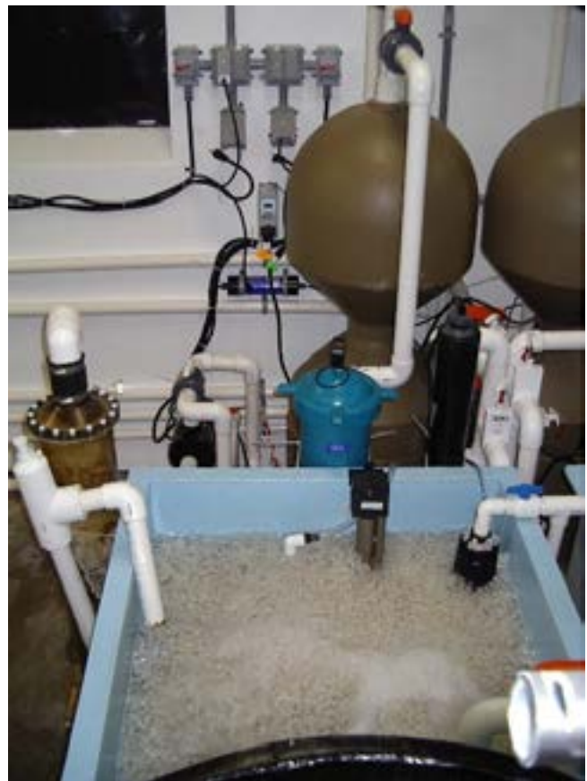
Fig. 1. RAS water treatment
